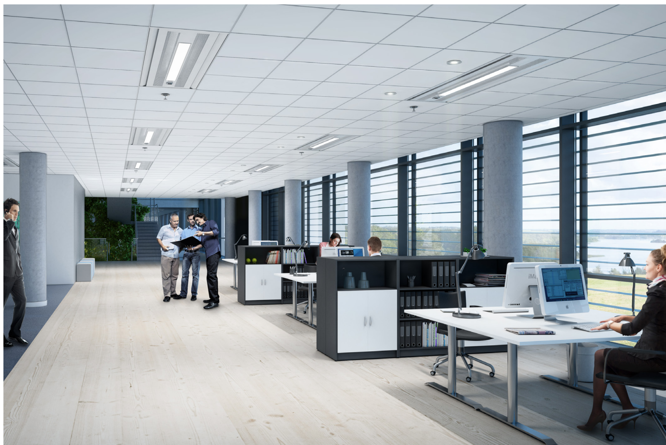
Picture 1. Open office, Professor active chilled beam installed with integrated lighting.
