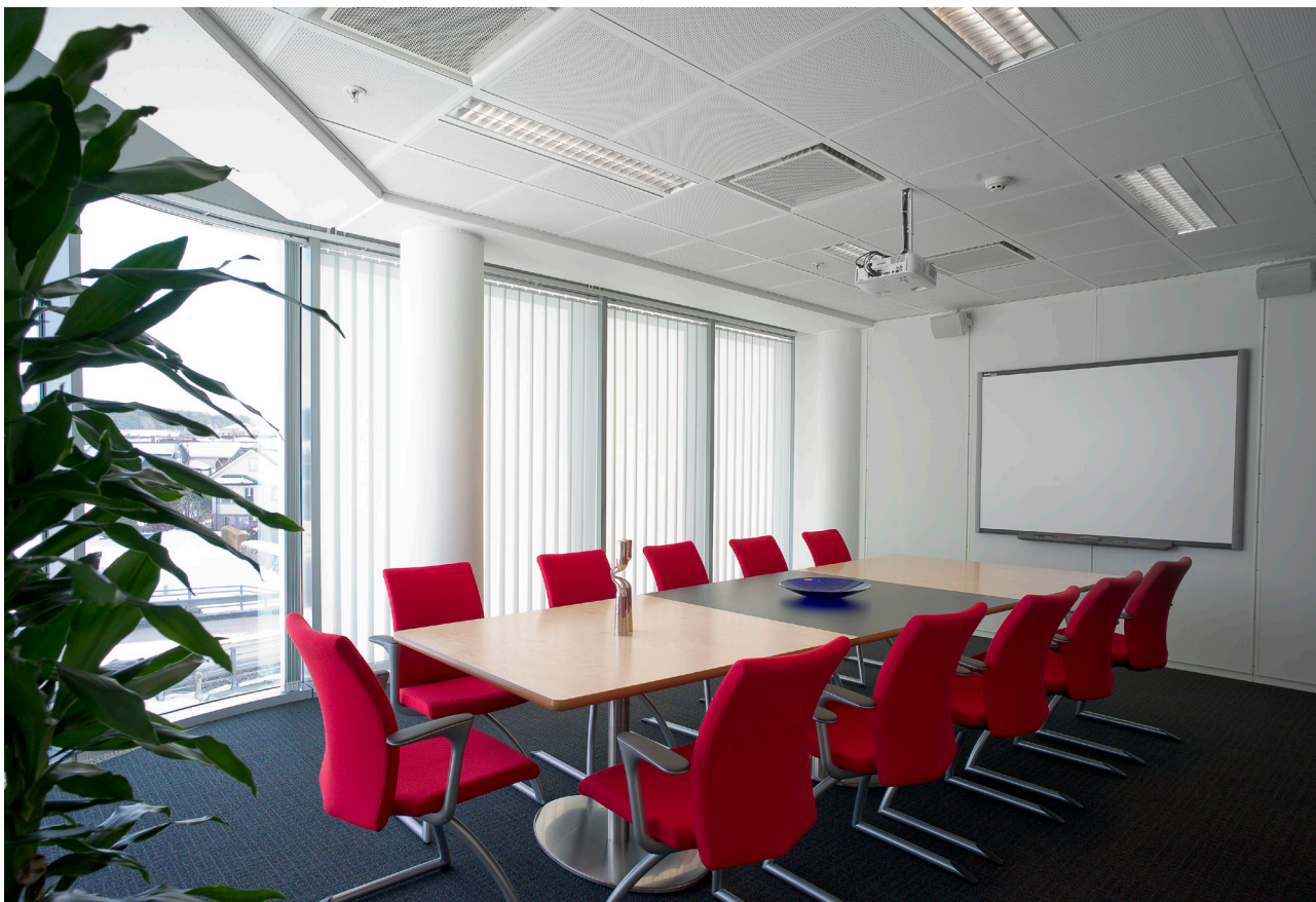
Picture 3. Meeting room, active chilled beams Plexus with separate regulated lighting.
