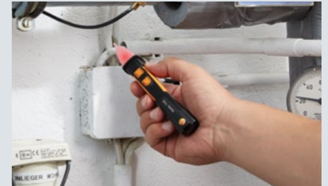
Non-contact voltage testing on a distributor box for a heating system with the testo 745.
